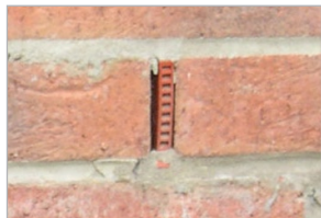
A badly installed 'weep vent'
